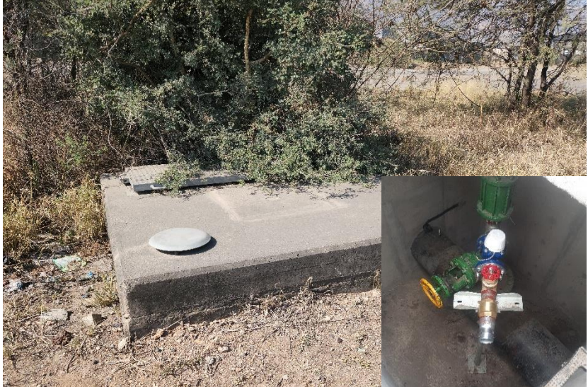
Water Source at Entrance
