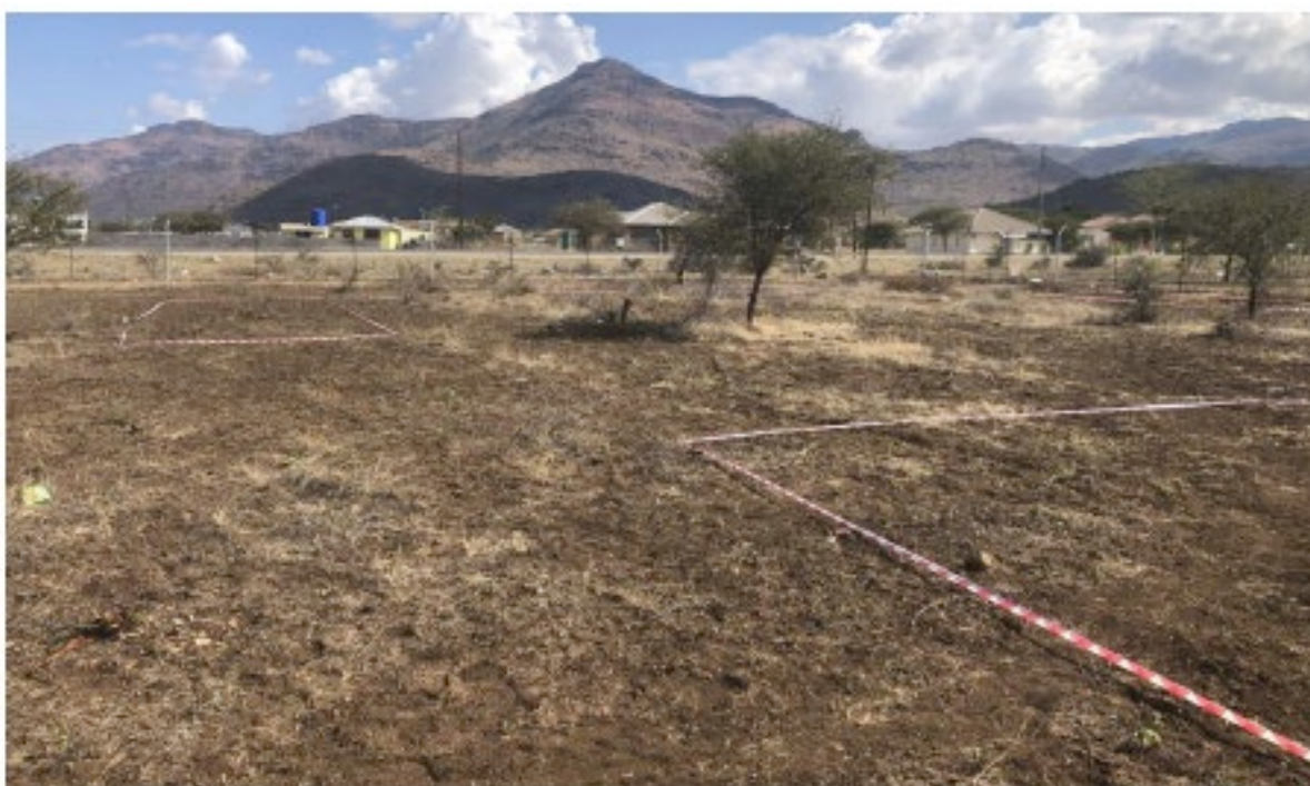
Contractor GeoMech has set out its laydown area to commence drilling within the newly-constructed security fence
