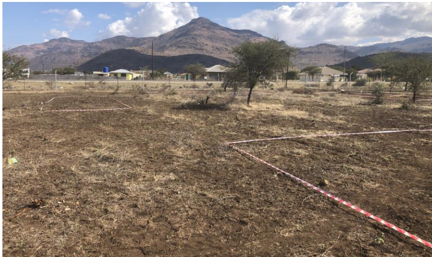
Drillers GeoMech have already set out their laydown area within the security fence.
